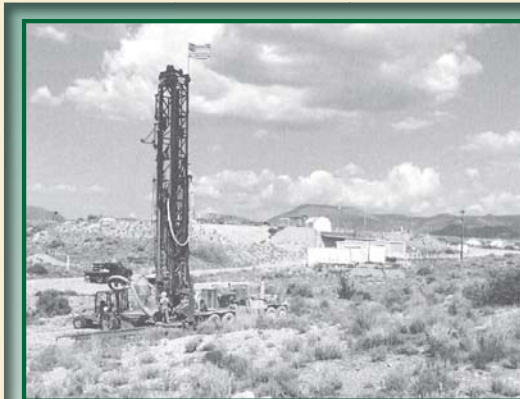
Drilling the borehole for groundwater monitoring well CTF-MW3 west of DSS SWMU 149 with Building 9930 in the background - 8/20/01. View looking northwest.
