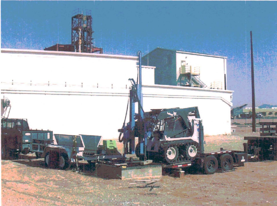
Figure 3.3-2 Soil sampling with the Geoprobe™ at the Building 6536 southwest seepage pit. View to the north toward Building 6536. September 4, 2002
