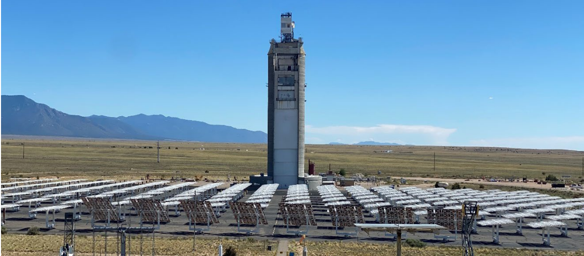
Figure 1: Heliostat field and central solar tower at Sandia's NSTTF with solid particle receiver mounted on top of the tower.
