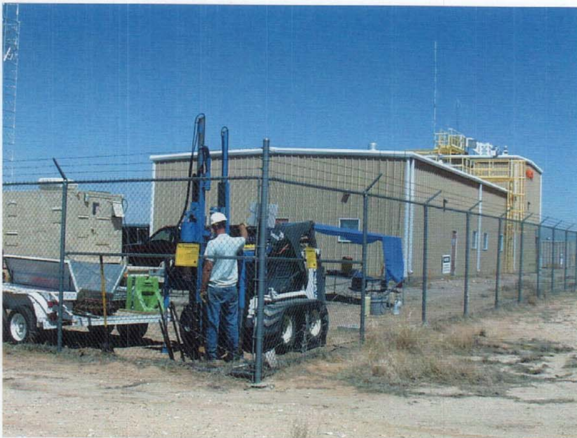
Figure 3.4-1 Collecting soil samples with the Geoprobe™ from the borehole through the drywell at DSS Site 1120, the Building 6643 Drywell. View to the northwest. August 22, 2002
