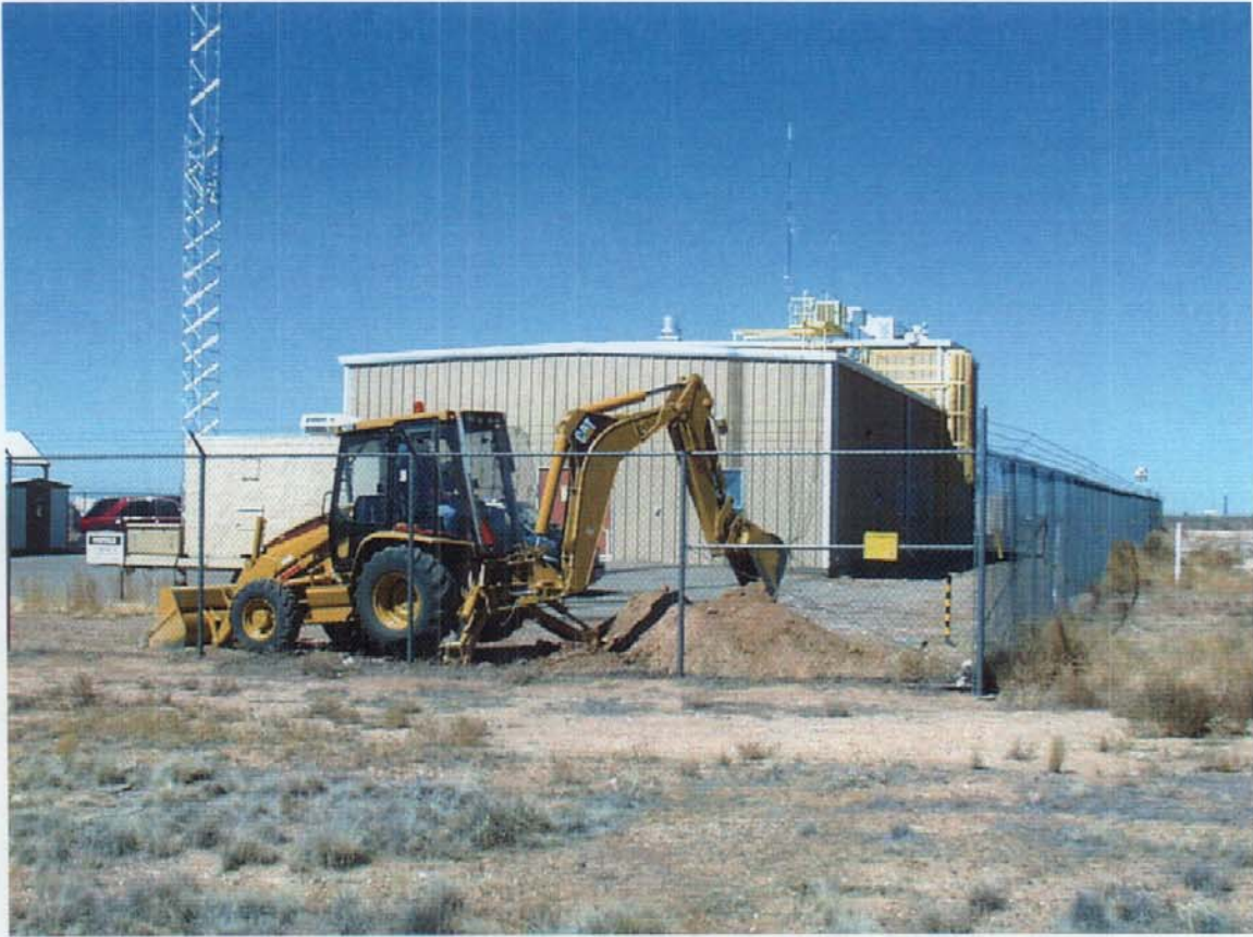
Figure 3.2-1 Backhoe excavation of DSS Site 1120, the Building 6643 Drywell. View to the northwest. March 20, 2002
