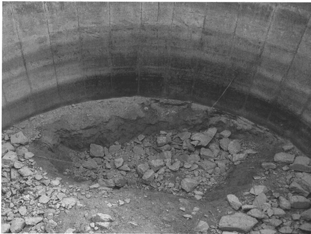
Figure 2. The wall debris was knocked into the bottom of the Cistern.
