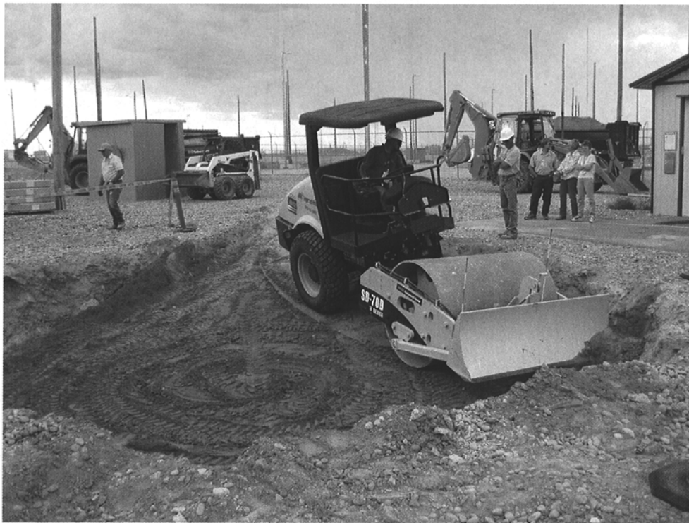
Figure 4. The backfill soil was compacted starting at approximately 3-4 feet below ground surface and continuing in 1 foot lifts to the ground surface.
