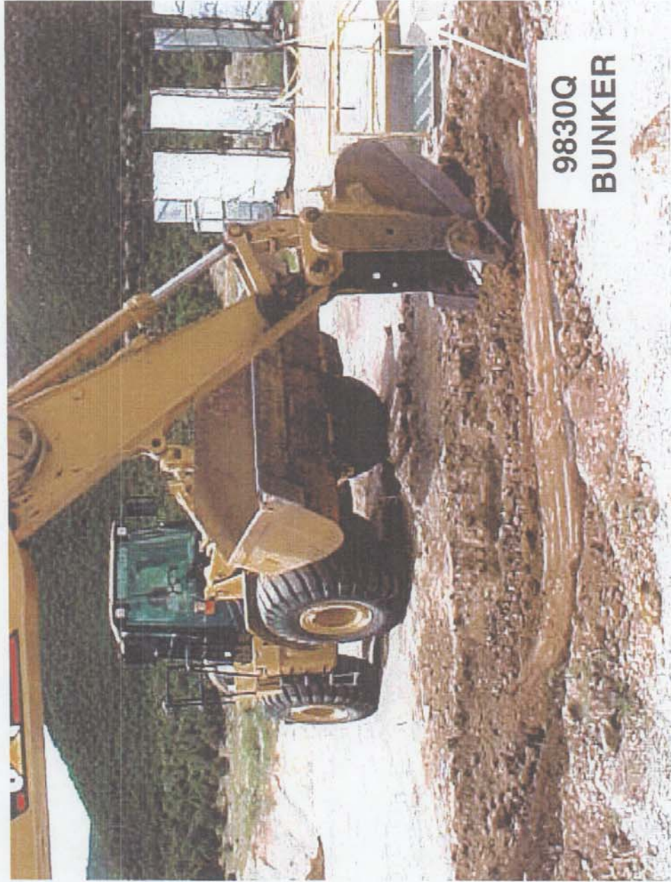
Figure 3.4.6-1 Removing Clean Soil Overlaying the Conduit Piping System (view to the southeast)
