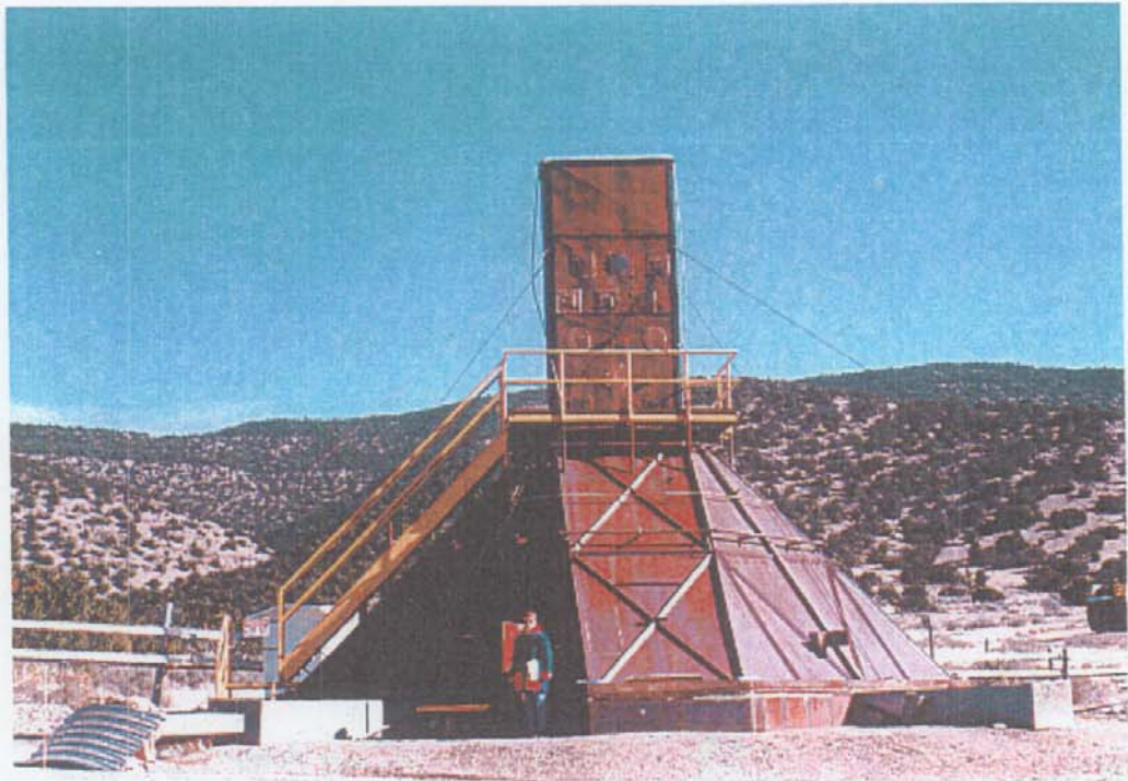
Photograph of the SWISH Unit at SWMU 94 in December 1994. View is to the north.
