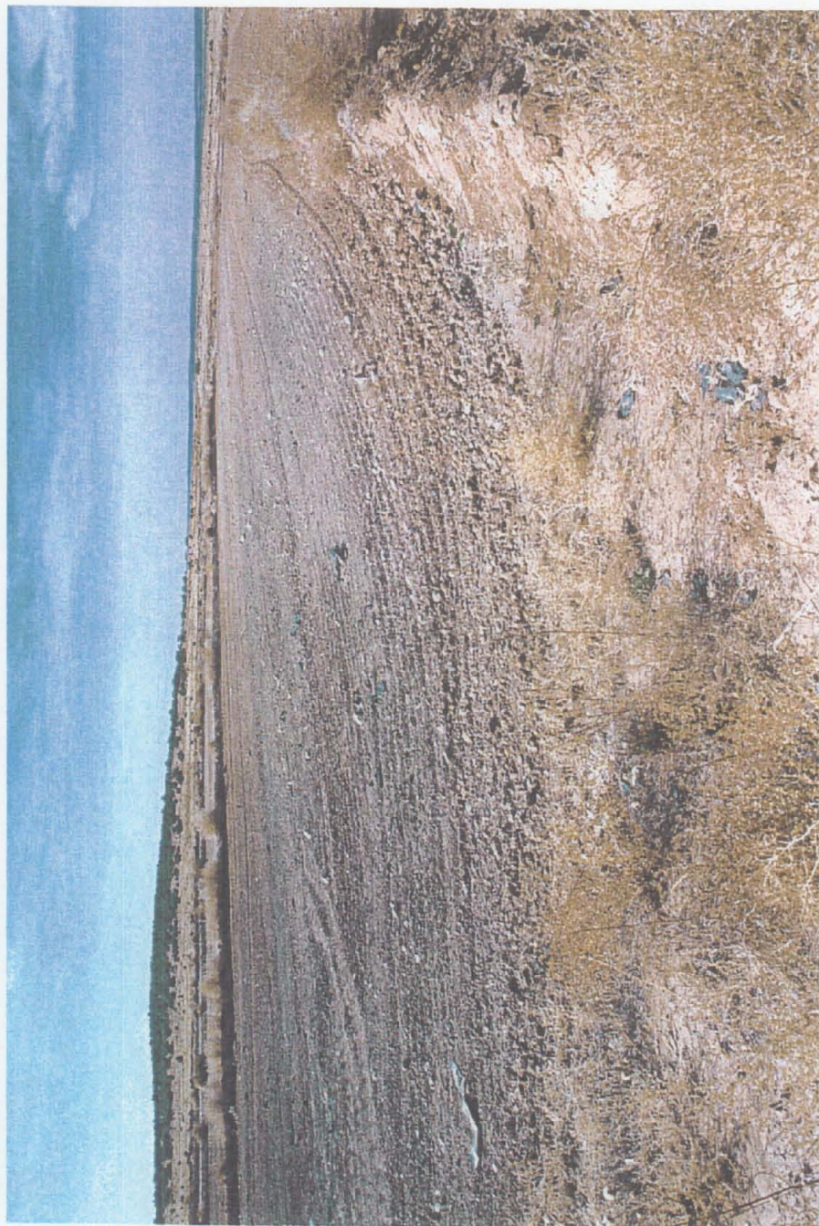
Figure 3.4.6-14 SWMU 94H Fuel-Contaminated Soil in Treatment Cell At KEERS Landfarm (view to the east)
