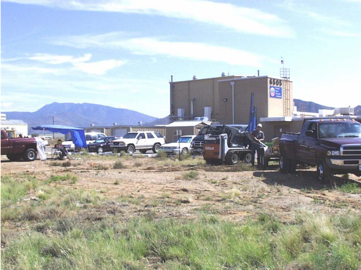
Figure 3.5-1 Collecting soil samples with the Geoprobe™ from beneath DSS Site 1084, Building 6505 Septic System drainfield. View to the northeast. August 20, 2002
