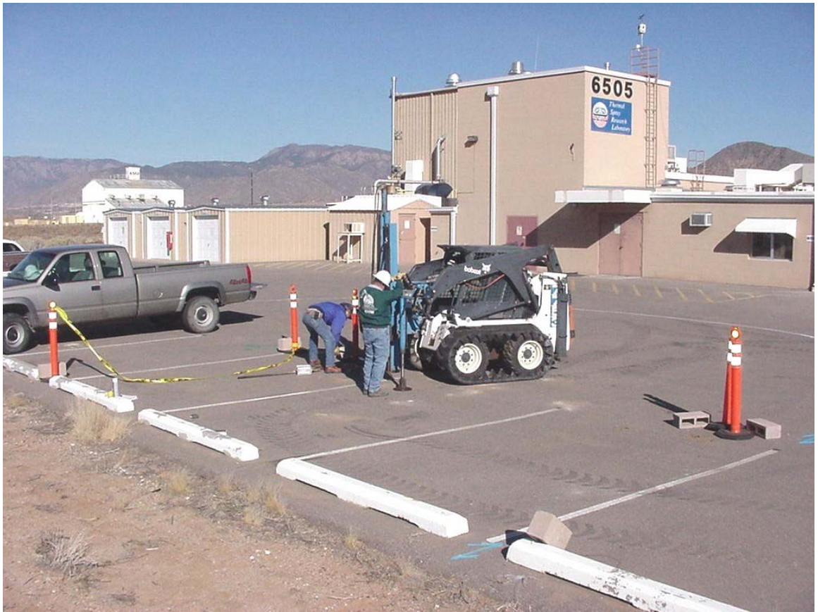
Figure 3.6-1 Using the Geoprobe™ to determine the location of the DSS Site 1084 septic tank, which was located beneath the asphalt pavement. View to the northeast. December 4, 2003
