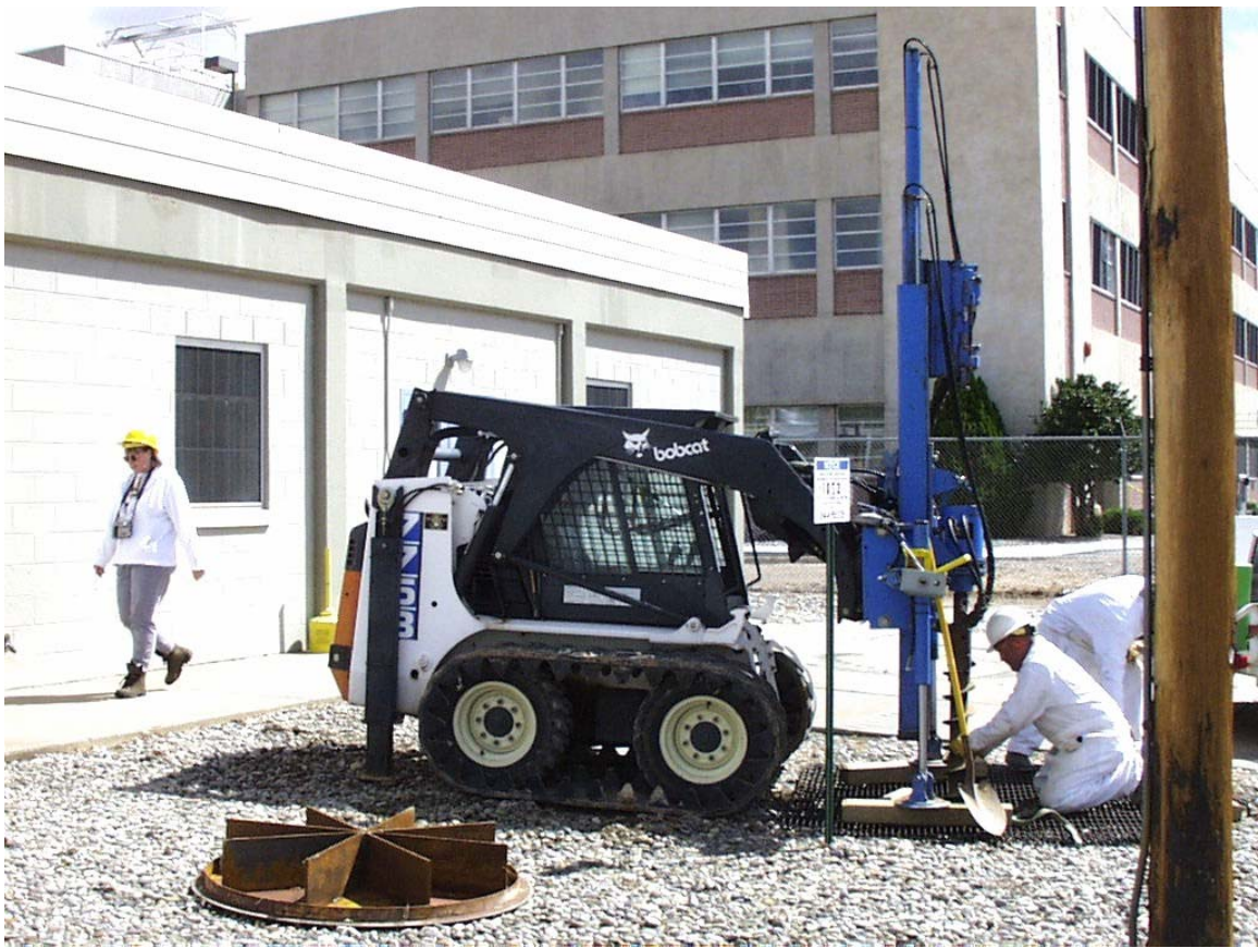
Figure 3.3-1 Collecting soil samples with the Geoprobe™ from the borehole drilled at DSS Site 1052, the Building 803 Seepage Pit. View to the southeast. September 19, 2002
