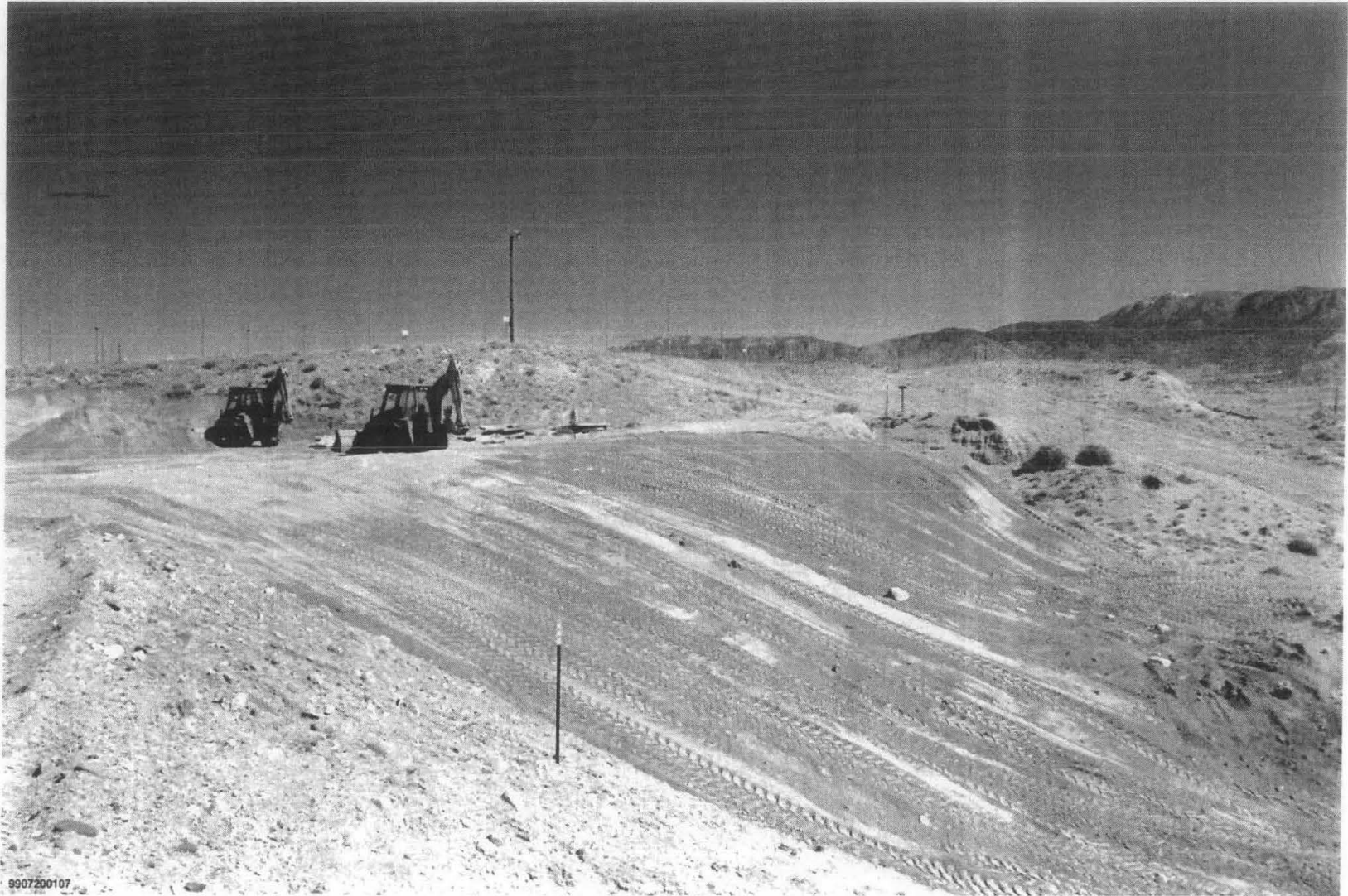
Figure 3.4.5-6 March 1999 photograph of the northern end of SWMU 228A after completion of the confirmatory work. A pair of backhoes are restoring the natural grade.
