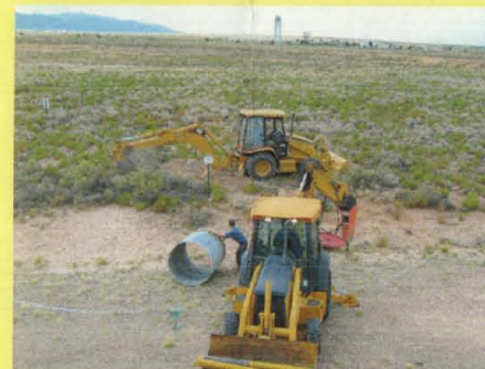
Backfilling the seepage pit excavation at AOC 1095. The section of metal culvert that was removed from the seepage pit is next to the worker in the foreground. The Solar Tower is in the background.
