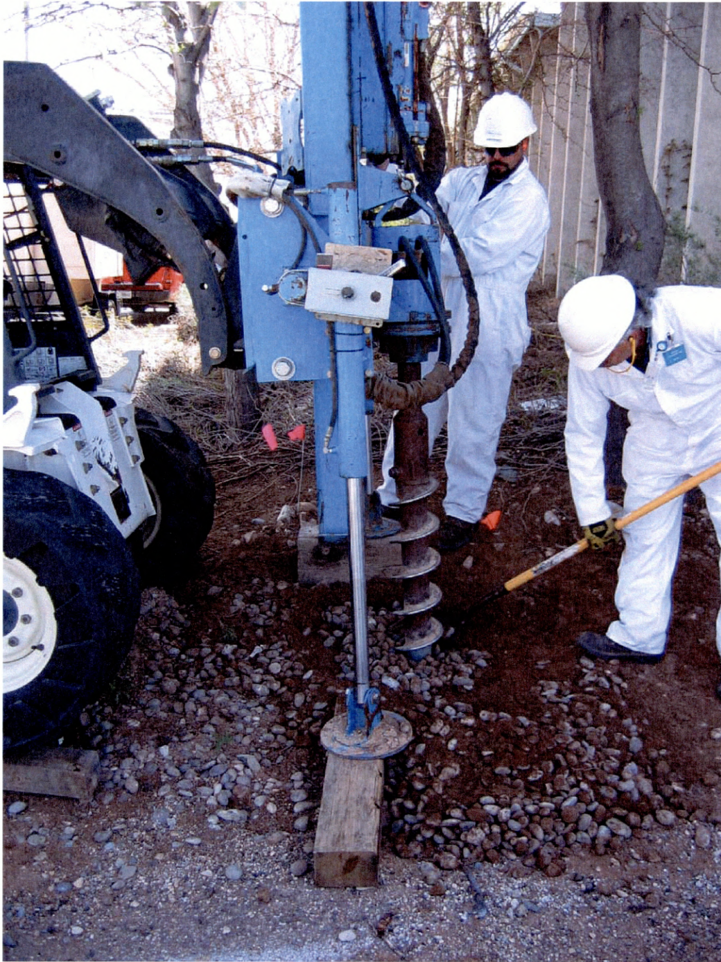
Figure 3.2-1 Auger drilling through the gravel aggregate to collect additional soil samples for VOC analysis at DSS Site 1117, the Building 9982 Drywell at the Solar Tower Complex. View to the east. April 14, 2005
