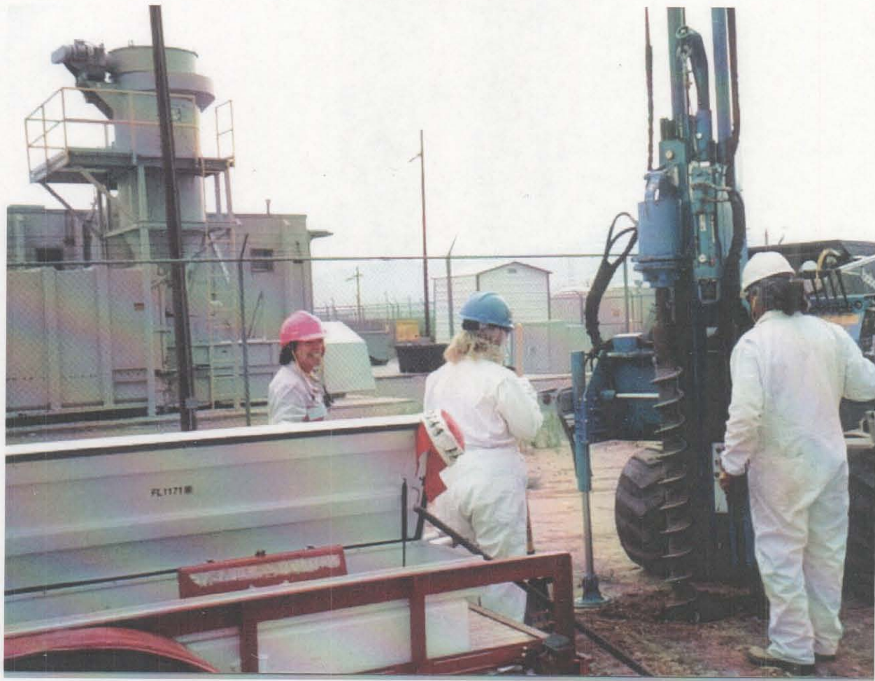
Figure 3.4-1 Collecting soil samples with the Geoprobe at DSS Site 1093, Building 6584 west septic system drainfield area. View to the northeast. August 19, 1999
