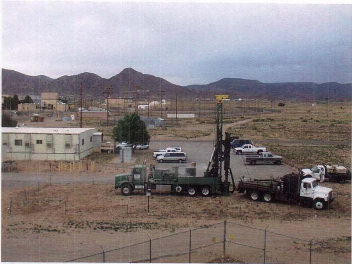
Figure 3.5.2-1 Borehole drilling for FLUTe™ soil-vapor monitoring well 1092-VW-01 in the MO 228-230 drainfield. The MO 228-230 complex is in the left-center of the photograph. View to the east. June 9, 2003
