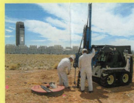
Collecting additional soil samples for VOCs from a borehole drilled adjacent to the seepage pit at AOC 1116 with the Solar Tower in background.
