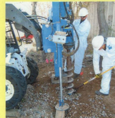
Auger drilling through the gravel aggregate to collect additional soil samples for VOC analysis at the AOC 1117 Drywell.
