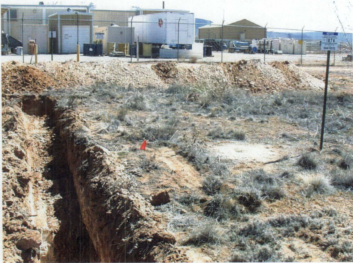
Figure 3.3-1 Backhoe excavations in the Building 6640 Septic System drainfield area to determine the locations and depths of the DSS Site 1078 drain lines. View to the southeast. March 18, 2002
