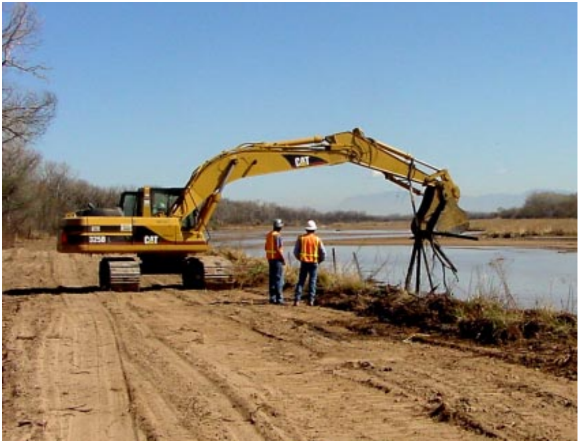
Fig. 17: Los Lunas, west bank. The first day of jetty jack removal, Apr. 9, 2002. Bankline jacks are the first to be removed. The job of removing 1,355 jacks is expected to take one to several months. Photo by Mark Horner, U.S. Army Corps of Engineers.
