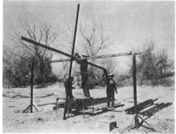
Fig. 3: Workers assemble a jack on site. Casa Colorado area, Middle Rio Grande Project, NM. Photo:Herman E. Carter, Bureau of Reclamation (Carlson and Enger 1956).
