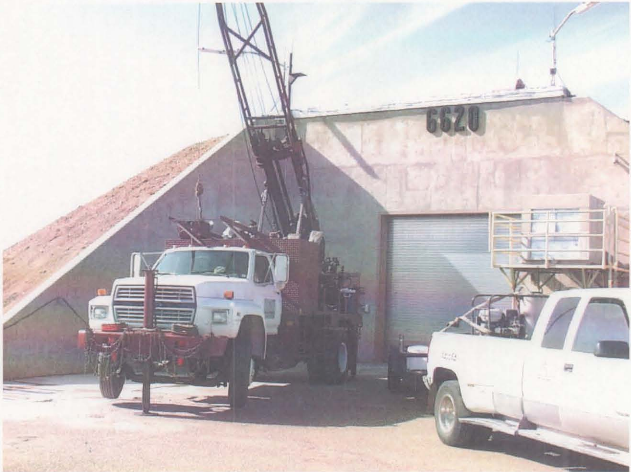
Figure 3.2-1 Auger rig set-up in preparation to drill an angled borehole beneath DSS Site 1009, the Building 6620 internal sump, from outside Building 6620. View to the northwest. November 1, 2002
