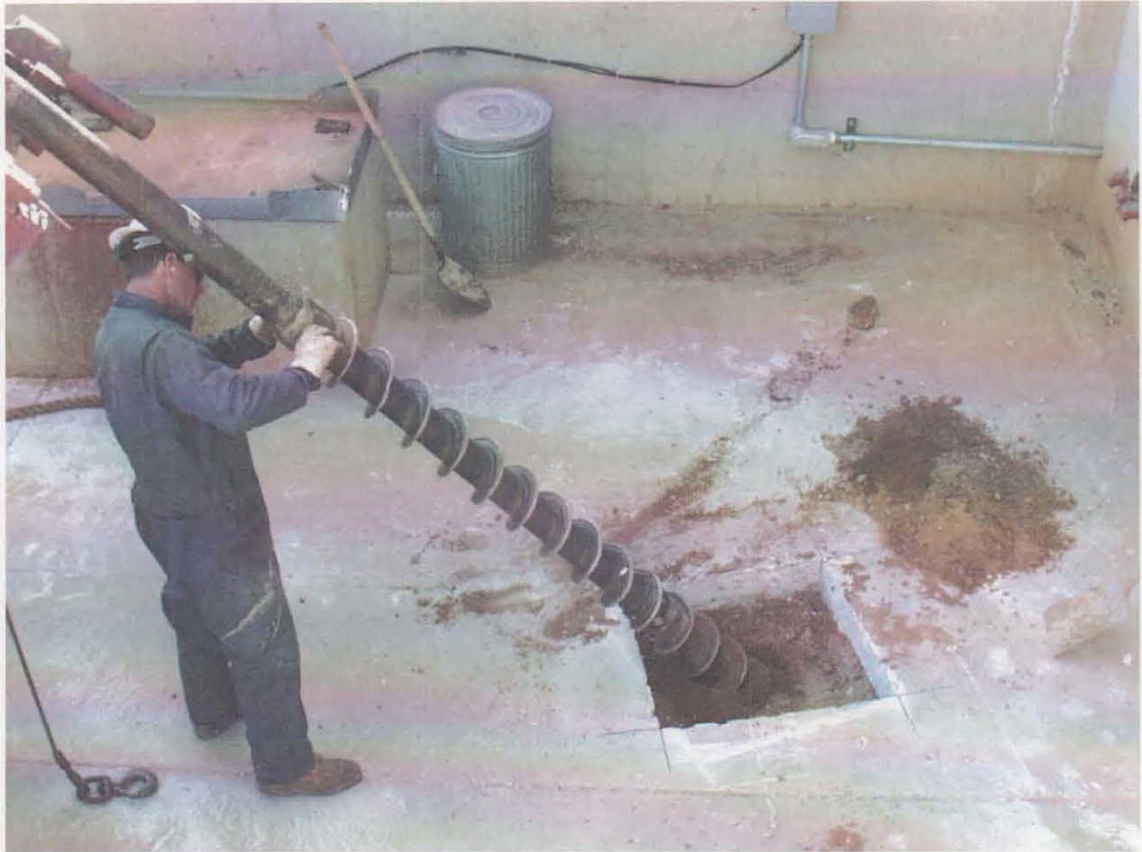
Figure 3.2-2 Drilling an angled borehole through the concrete slab on the south side of Building 6620 to collect soil samples from beneath DSS Site 1009, Building 6620 internal sump. View to the southwest. November 1, 2002
