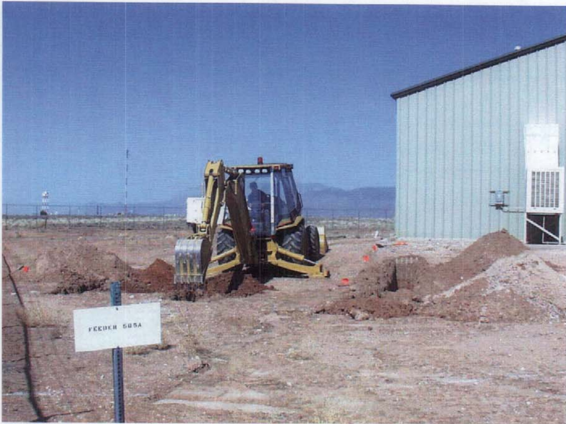
Figure 3.4-1 Exploratory backhoe excavation to locate the DSS Site 1080 septic system drainfield drain lines at Building 6644. View to the north. March 14, 2002
