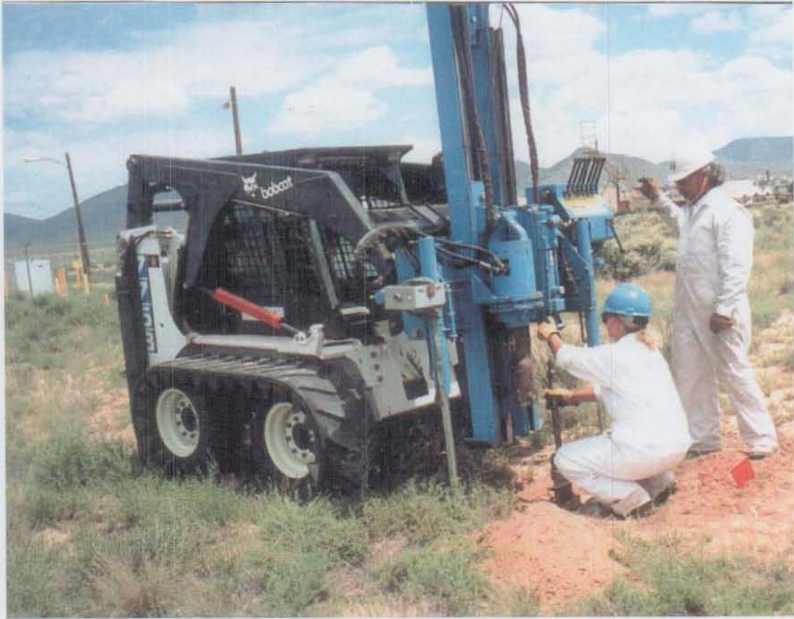
Figure 3.4-1 Collecting soil samples with the Geoprobe™ at DSS Site 1006, the Building 6741 drainfield. View to the northeast. August 18, 1999
