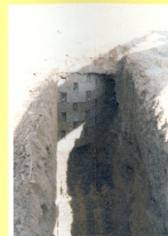
This is a partially excavated seepage pit at DSS SWMU 159. This seepage pit is constructed of unmortared concrete blocks and was surrounded by a layer of gravel. Seepage pits like these typically had several feet of gravel in the bottom. The seepage pit is approximately 7 ft deep and 5 ft in diameter. The inlet pipe is approximately 5.5 ft below grade.
