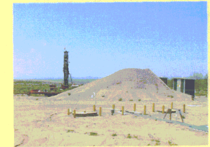
Drilling groundwater monitoring well CTF-MW2 northwest of SWMU 154 with the two HE seepage pits and an HE storage bunker in the foreground.
