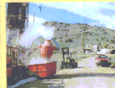
Drilling groundwater monitoring well CTF-MW1 southwest of SWMU 116. Drilling groundwater monitoring well CTF-MW2 northwest of SWMU 154 with the two HE seepage pits and an HE storage bunker in the foreground.
