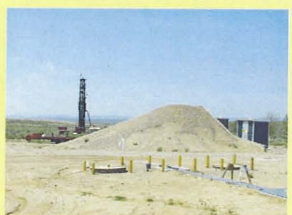
Drilling groundwater monitoring well CTF-MW2 northwest of SWMU 154 with the two HE seepage pits and an HE storage bunker in the foreground.
