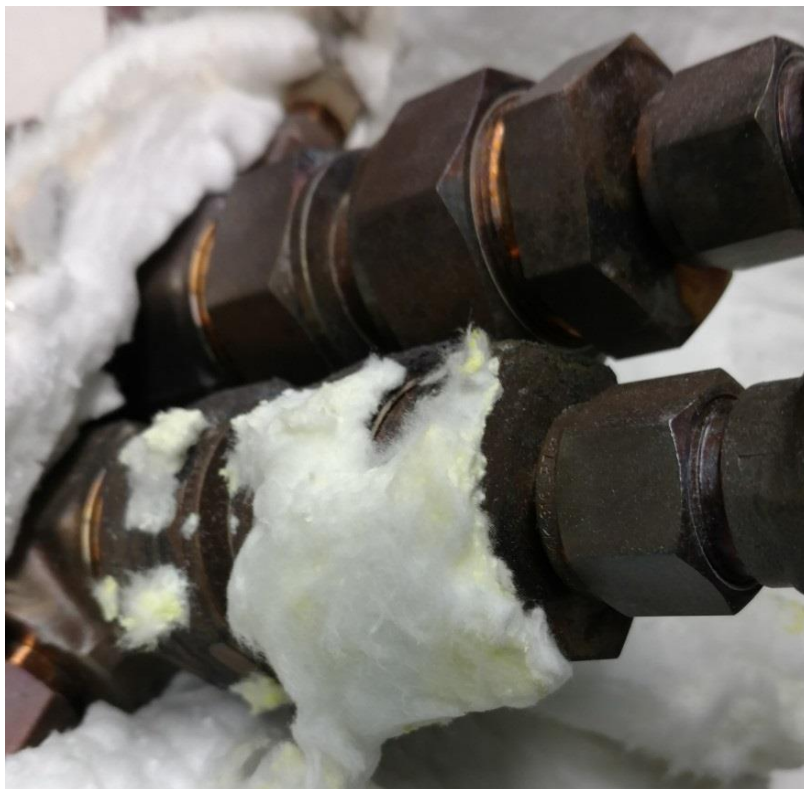
Figure 3-28 Pump outlet loop leg salt leak site
