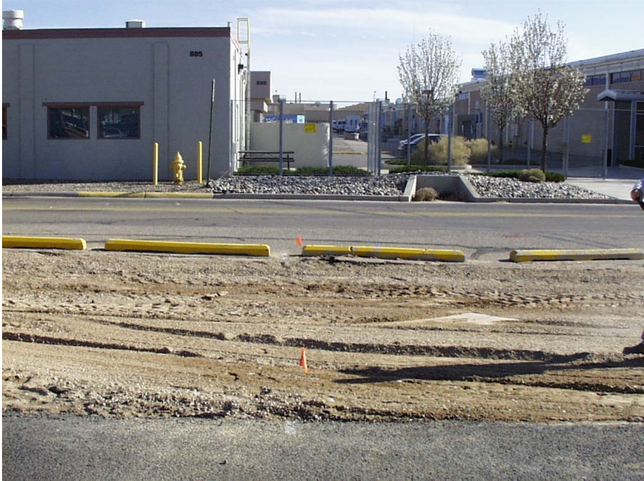
Figure 3.2-1 Two orange pinflags mark the location of the DSS Site 1101, Building 885 septic system, drain line running north from Building 885 (upper left of photo) and beneath "H" Street. View to the south. March 26, 2002
