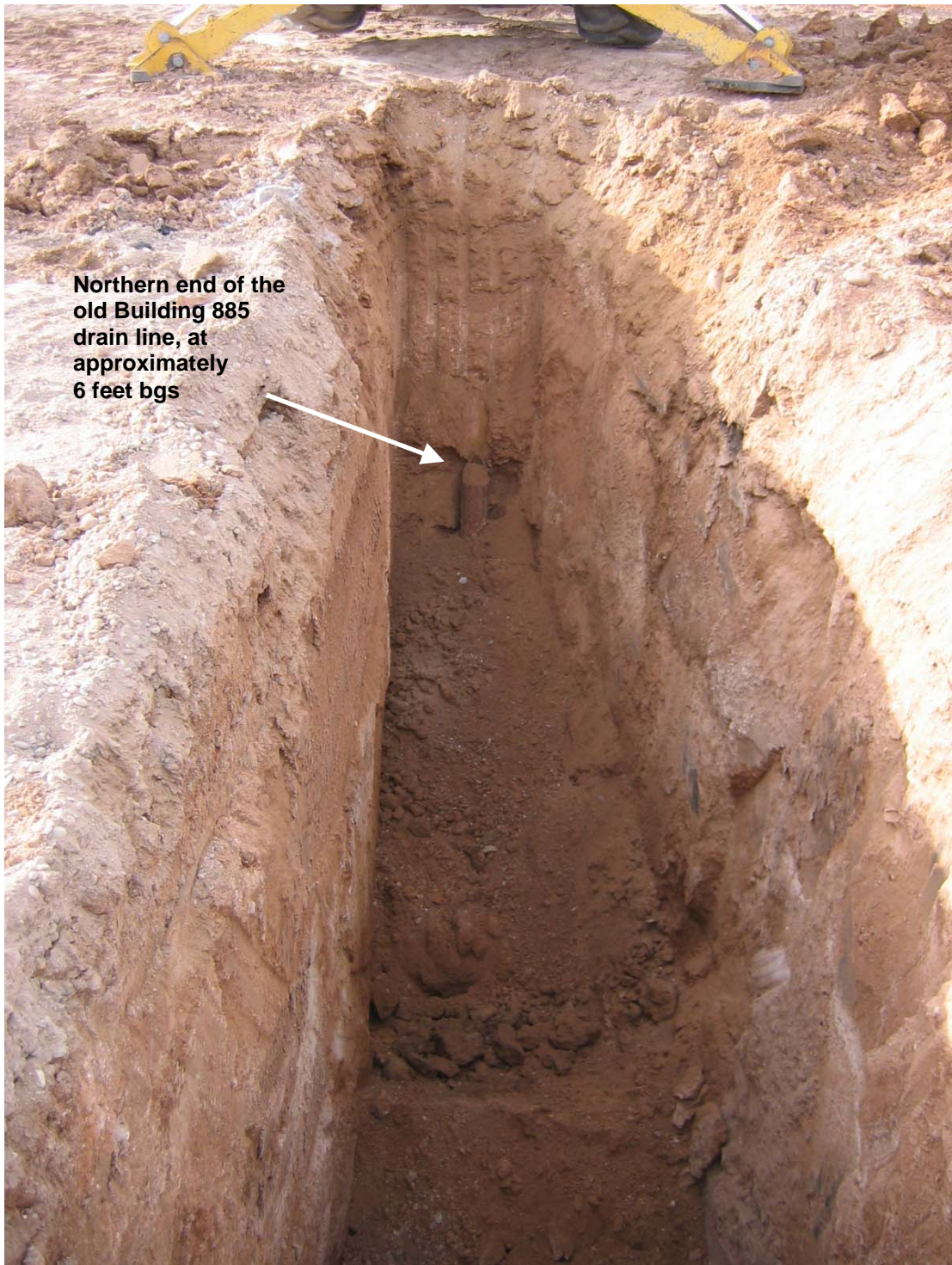
Figure 2-2 Excavation #3 showing the broken northern end of the old drain line running north from Building 885 and which marks the presumed location of the southern end of the former septic tank. View to the south. March 4, 2006.
