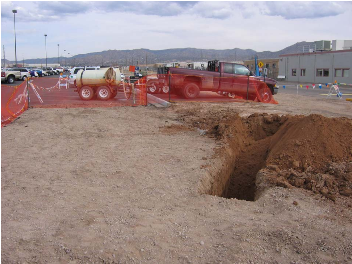
Figure 2-1 Backhoe Excavation #2 completed in the asphalt, curb, and gutter removal area at DSS Site 1101 to locate the buried drain line from Building 885. View to the southeast. March 3, 2006.
