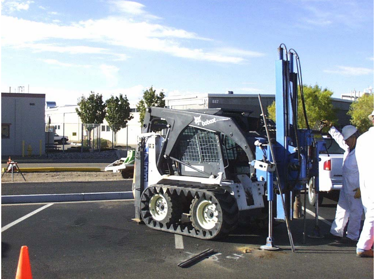
Figure 3.4-1 Auger drilling at the DSS Site 1101, Building 885 septic system seepage pit location in the parking lot north of Building 885, shown in the center-left side of the photo. View to the southwest. October 21, 2002
