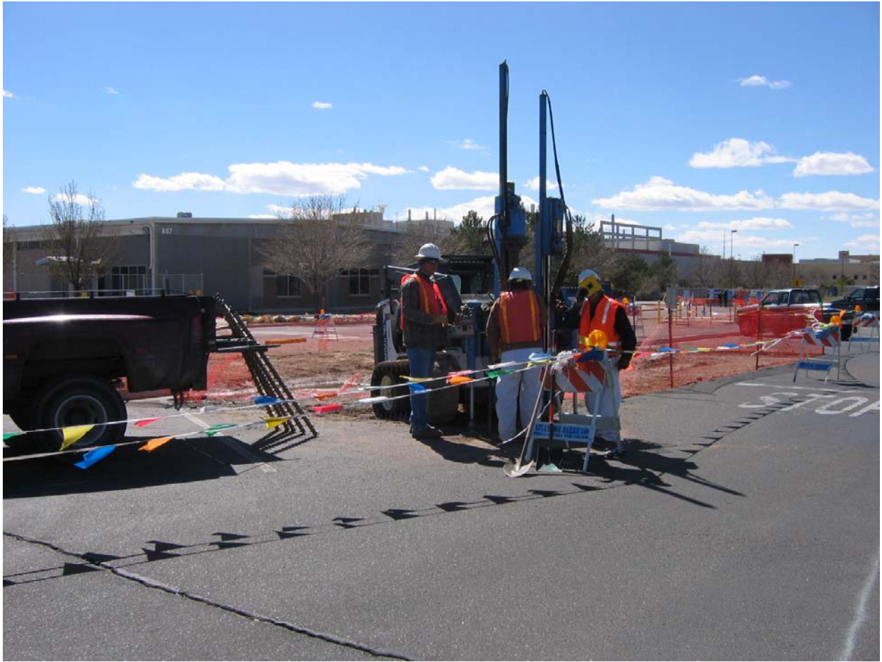
Figure 3-1 Collecting soil samples with the auger rig from beneath the center of the former northeast seepage pit location as indicated in engineering drawings. View to the southwest. March 13, 2006.
