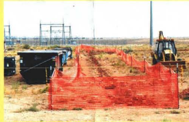
VCA remediation trench at SWMU 46. Roll-off bins for waste (contaminated soil and pipe pieces) are located along east side of trench. View to south, August 2003.
