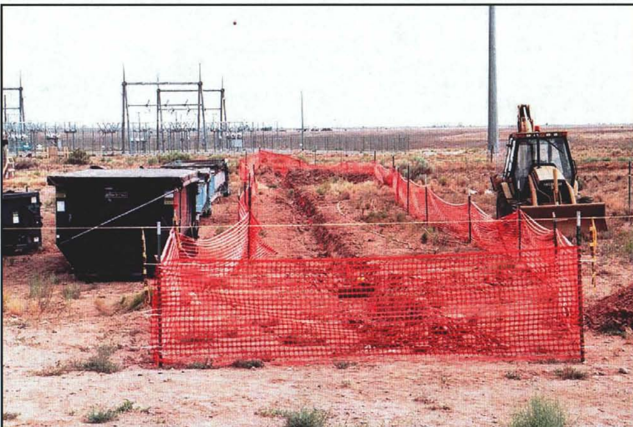
Figure 5 Handheld photograph showing the VCA remediation trench at SWMU 46. Roll-off bins for waste (contaminated soil and pipe pieces) are located along east side of trench. View to the south, August 2003.
