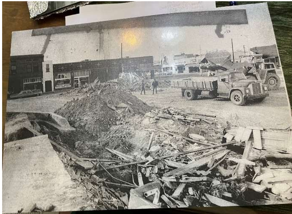
FIGURE 16 IMAGE OF THE DEMOLITION OF ST. GENEVIEVE'S CHURCH PHOTO PROVIDED BY IRENE OLIVER LOUISE AND DAVID CHAVEZ
