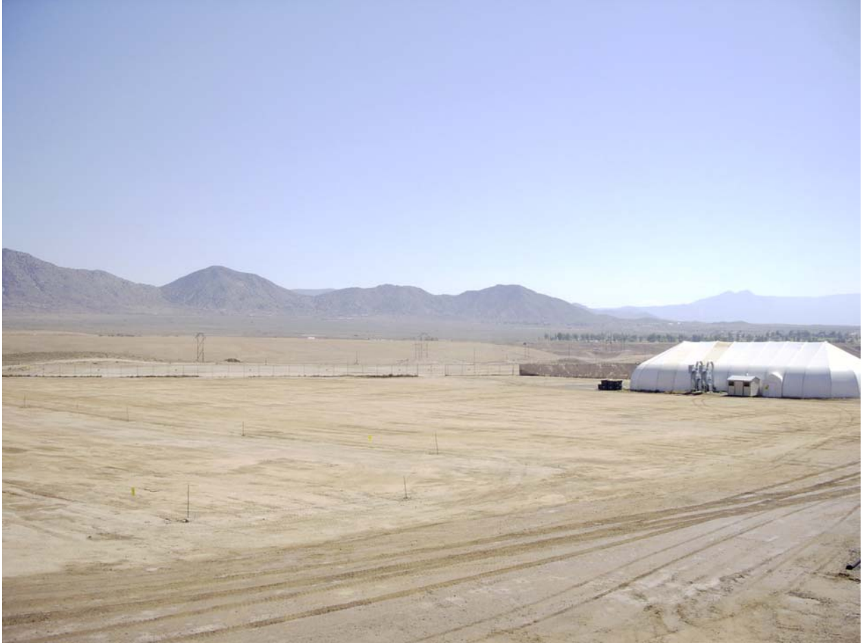
Figure 6-8 Classified Waste Landfill Excavation After Final Site Grading. View to the Southeast. September 29, 2003
