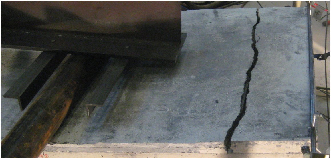
Figure 5.17: Horizontal shear failure of the UHPC overlay outside of the shear-friction reinforcement (plan)
