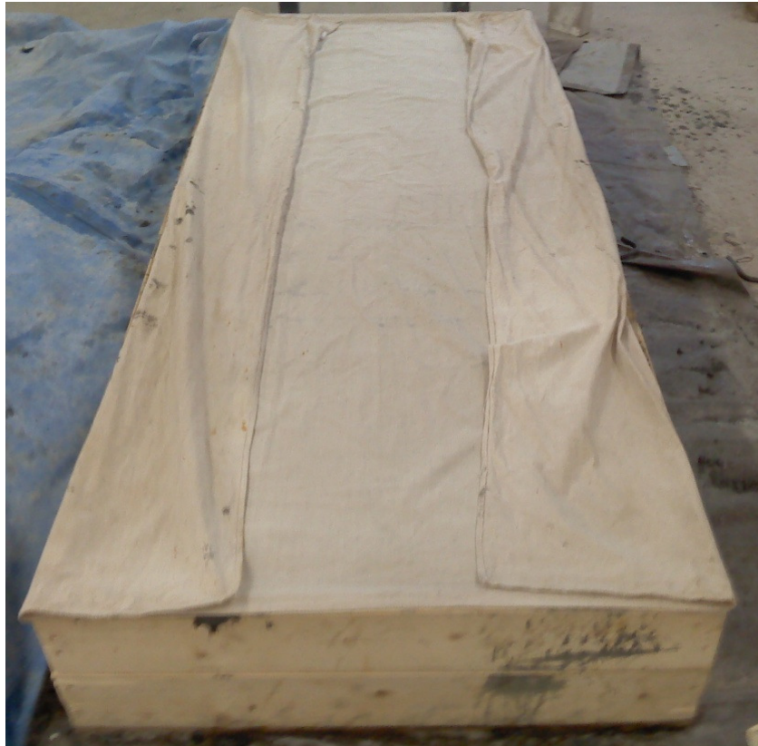
Figure 3.25: Canvas to prevent cracking during the initial set of the UHPC overlay
