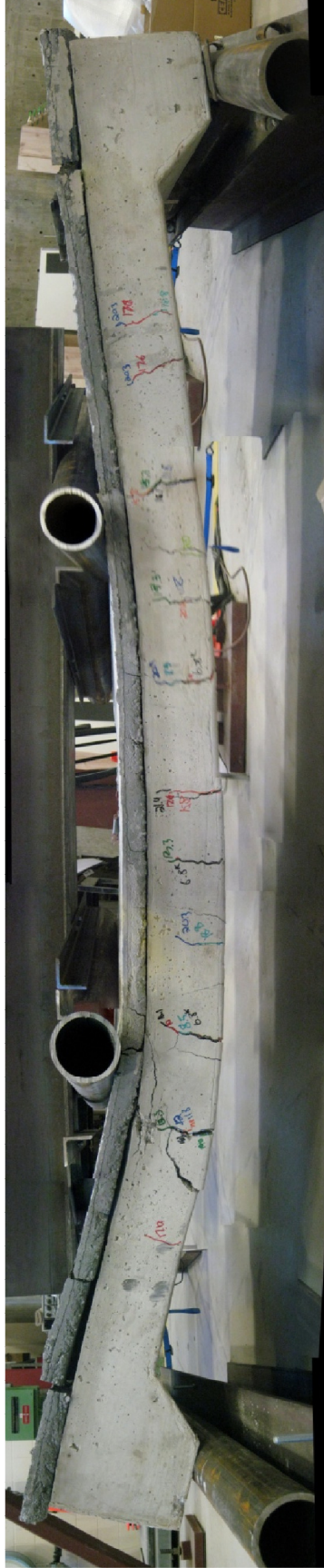
Figure 5.20: Profile of the strengthened slab at failure
