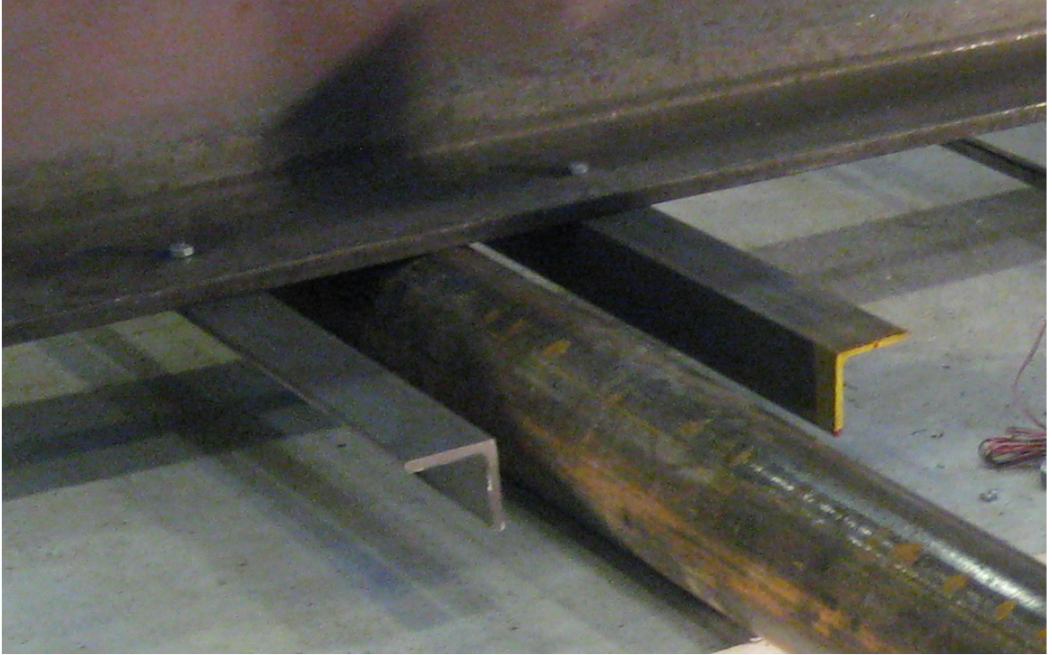
Figure 3.6: Angle iron used to restrict unexpected movement
