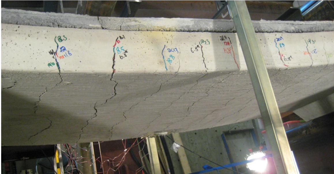
Figure 5.16: Flexural cracking of the strengthened concrete slab
