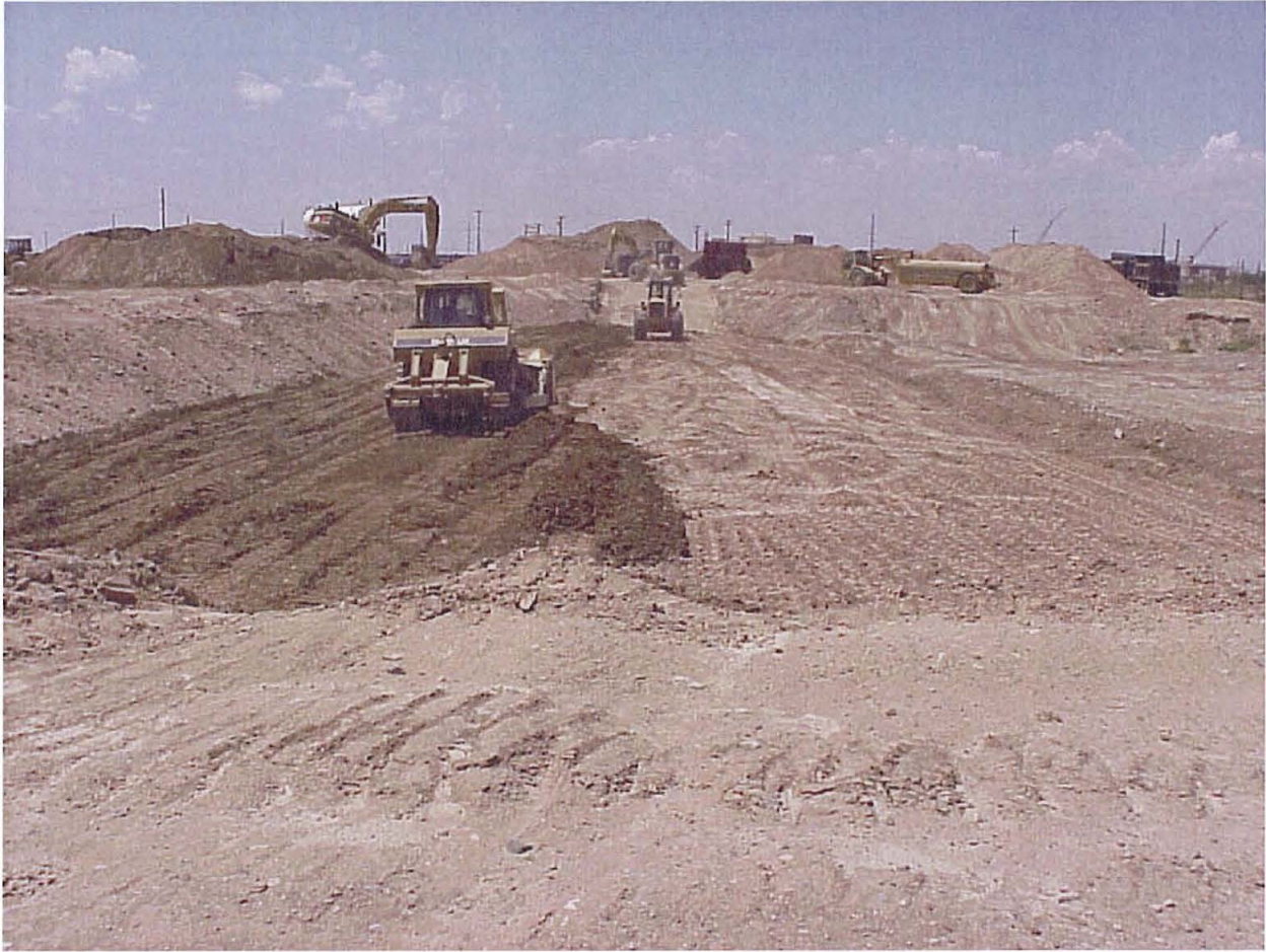
Figure 6.2-1 Photograph showing the SWMU 1 backfill operation on July 27, 2003. (The sheepfoot roller in the foreground is compacting Lift 8 at an approximate depth of 10 ft bgs. Heavy equipment in the background consists of excavators, loaders, a screen plant, a water truck, and a dump truck. View is to the northwest.)
