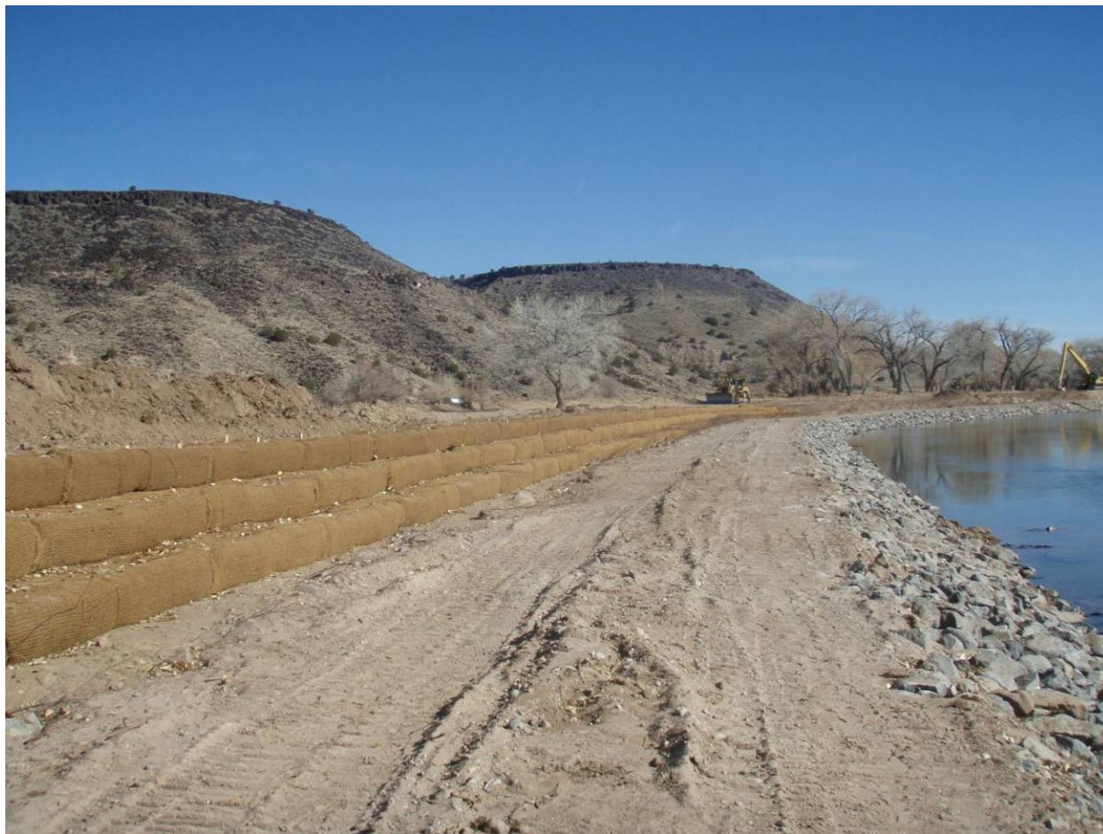
Photo 7: Rock toe and Bio-D blocks at Priority Site RM 213.4, San Felipe (February 2011, Benoit)
