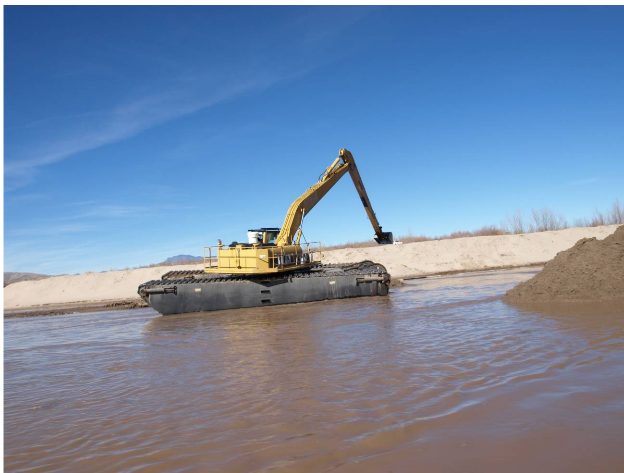
Photo 2: Amphibious excavator working on breach south of the Red Rock Staging Area (November 2010, Holste)
