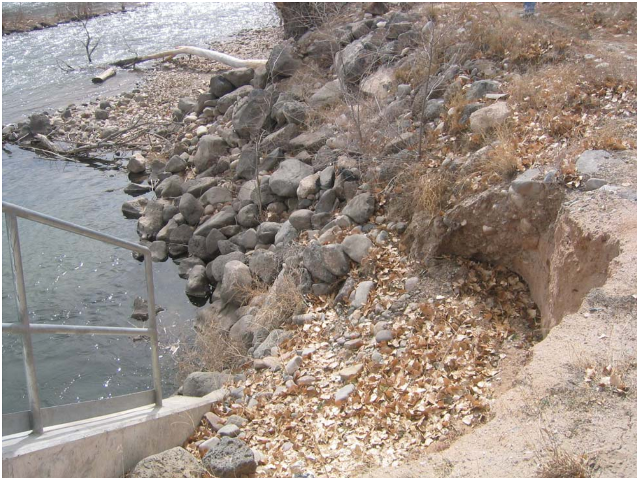
Photo 4: Looking down at the bank erosion on the south side of the Lyden outfall facility (March 2006)
