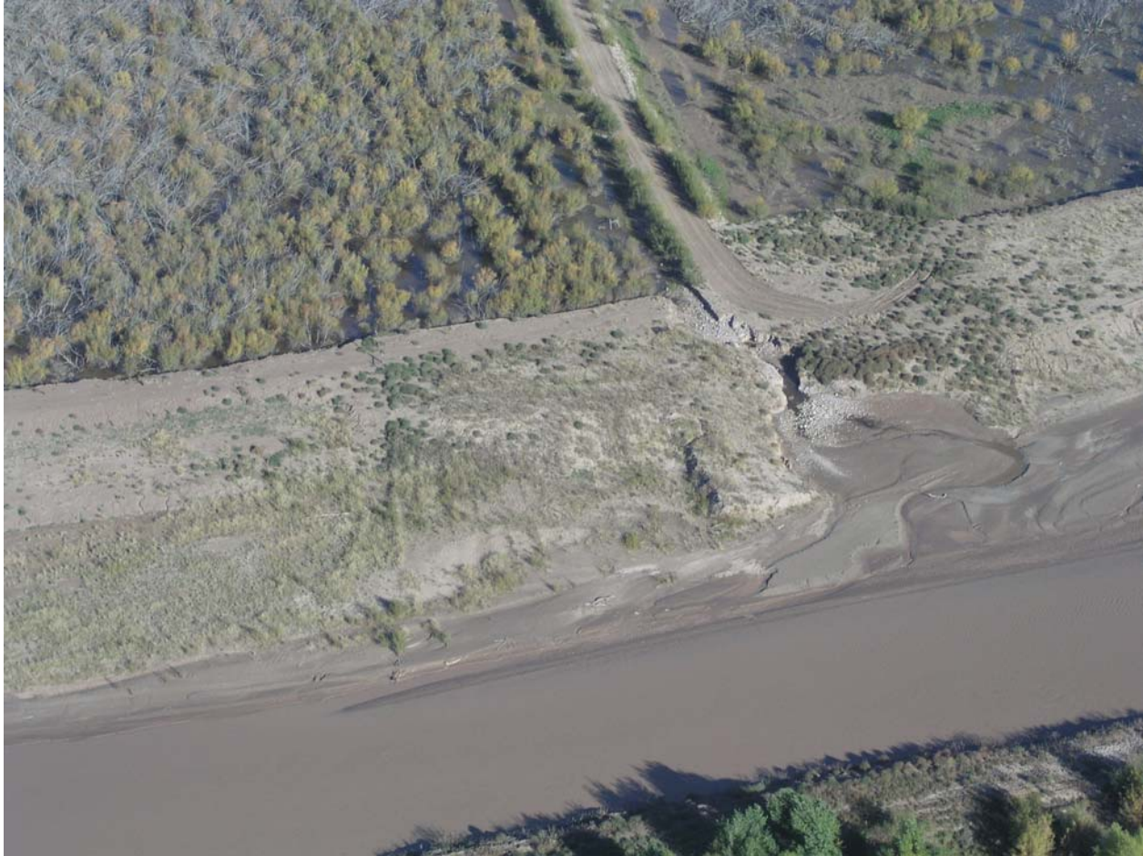
Photo 3: Temporary Channel 2000—berm breach at Nogal Canyon (October 2006)
