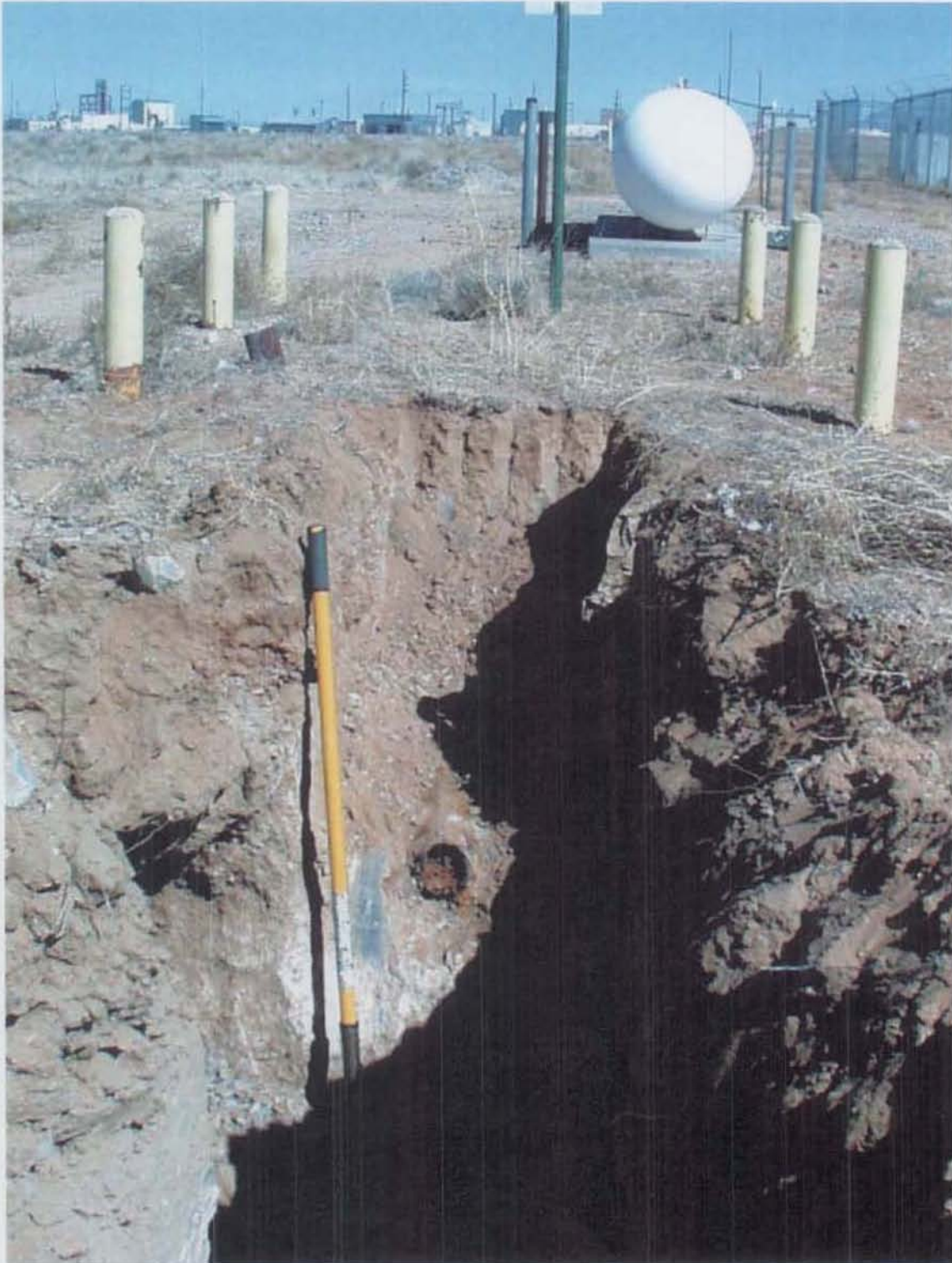
Figure 3.3-2 DSS Site 1083, Building 6570 drywell. The end of the 4-inch, cast iron drain pipe, which extended from septic tank to the drywell, is shown. View to the north. March 11, 2002
