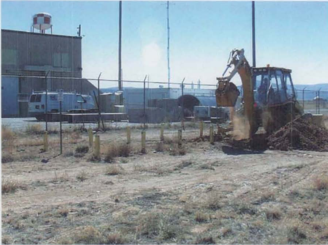
Figure 3.3-1 Backhoe excavation at DSS Site 1083, Building 6570. The drywell was located between the yellow posts. View to the southeast. March 11, 2002
