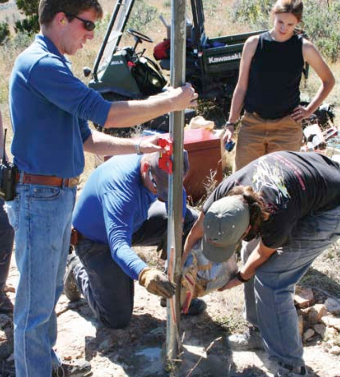
Technicians and engineers set a metal pole in concrete to support an equipment enclosure containing global positioning satellite wiring and electronics designed to measure the movement of the Rio Grande Rift. Photo by Steve Carr.
