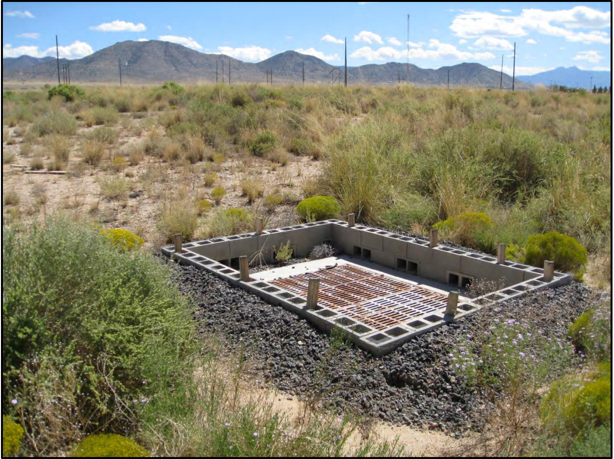
Figure 4: A typical block and gravel (B&G) inlet protection control structure used within the SNL MS4 to prevent trash and sediment from entering the stormdrain system.
