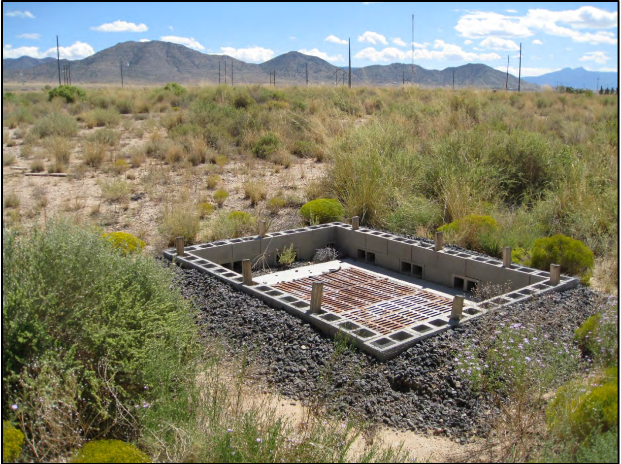
Picture of a typical "Block and Gravel" inlet protection control structure used at SNL/NM to prevent trash and sediment from entering the stormdrain system.
