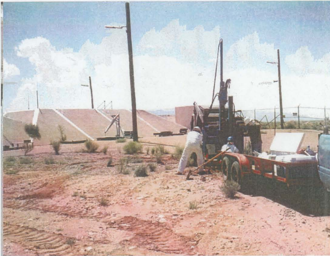
Figure 3.4-1 Collecting Soil Samples with the Geoprobe™ from the Building 6750 Septic System Drainfield, DSS Site 1008, August 17, 1999
