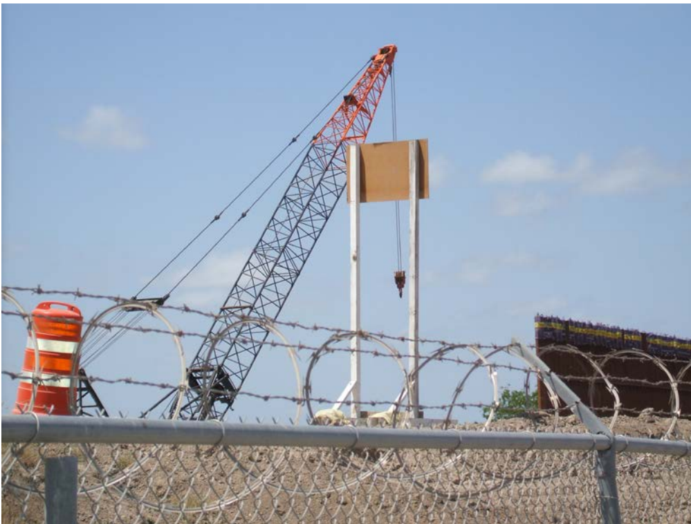
Figure 21: Border Wall under construction at Brownsville, Texas and Matamoros, Tamaulipas. Author photo.
