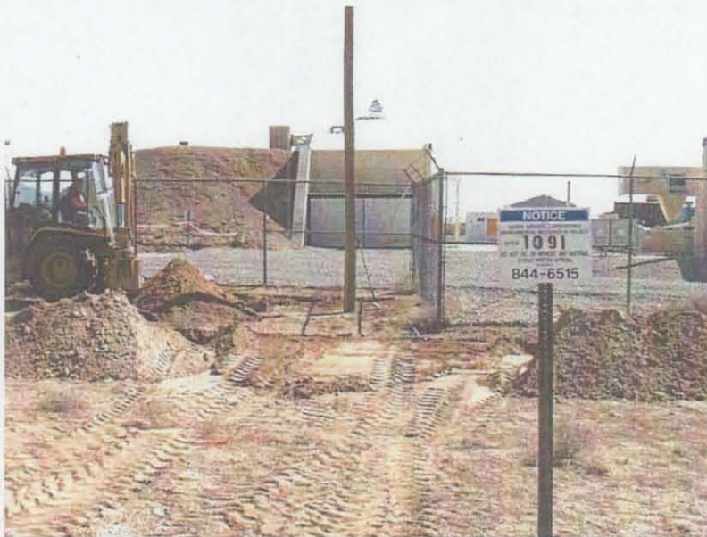
Figure 4-2 Trench Excavated at Septic Tank Location as Shown on Engineering Drawings North of Building 6720. Partly backfilled drainfield exploratory trench shown in Figure 4-1 is in the foreground. No evidence of a septic tank was found, and the septic system (DSS Site 1091) was determined not to exist. March 19, 2002
