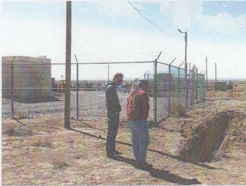
Figure 4-1 Trench Excavated East to West North of Building 6720 to Locate Possible Drainfield. No drainlines were found and the septic system (DSS Site 1091) was determined not to exist. March 19, 2002
