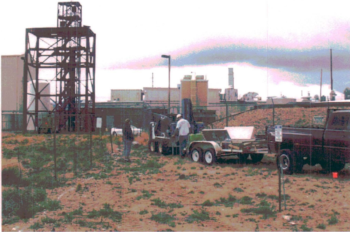
Figure 3.3-1 Collecting soil samples at DSS Site 1110, Building 6536 Drain System, with NMED Oversight Bureau regulator observing the process. View to the southeast. September 10, 2002
