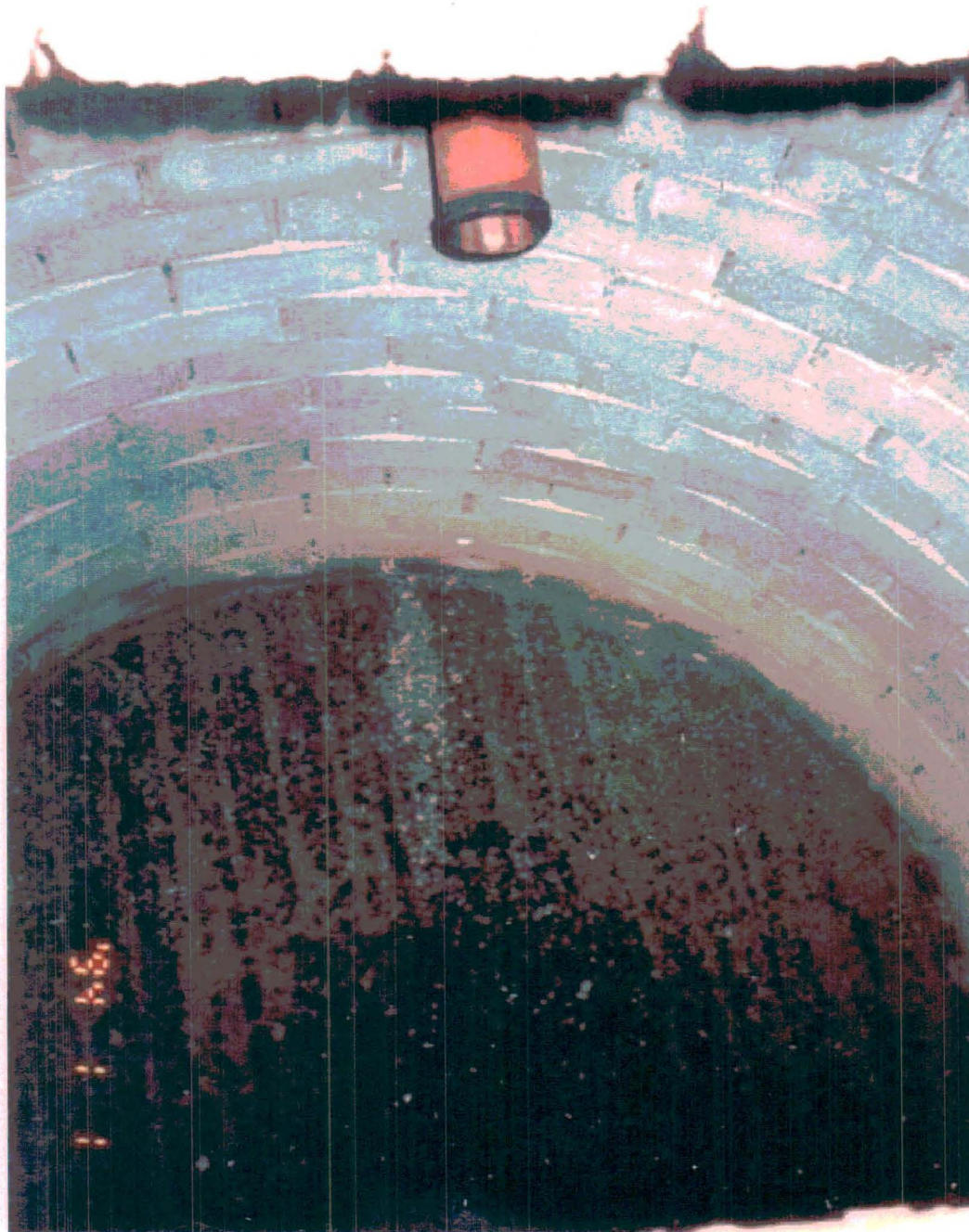
Figure 3.3-1 View into the interior of the single (southwest) seepage pit, constructed of stacked cinder block with an aggregate bottom, and with a drain line from Building 6536 at the top of the unit. July 16, 1999
