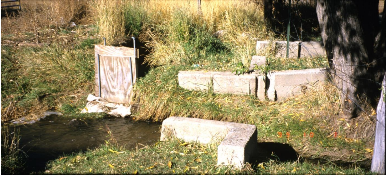
Compuerta to Lateral No. 2, October 1999
