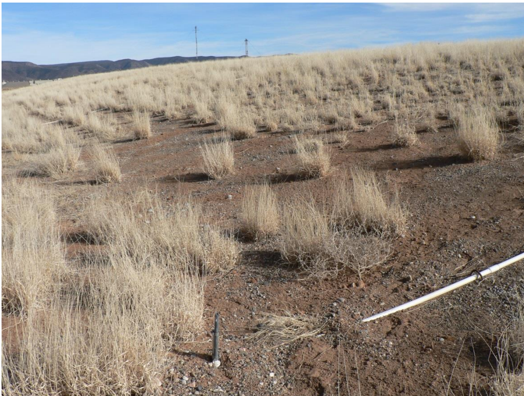
North slope of cover: facing east from the western portion of slope
