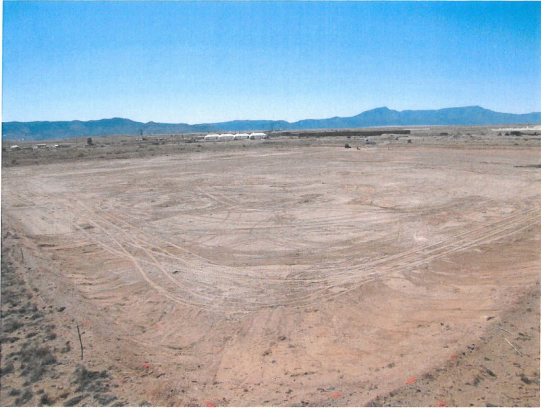
Borrow Pit in May 2013 at the start of the reclamation effort. View from northwest corner to southeast.
