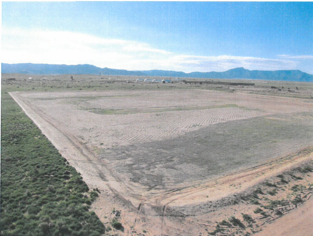
Borrow Pit in August after completion of the reclamation effort. View from northwest corner to southeast.
