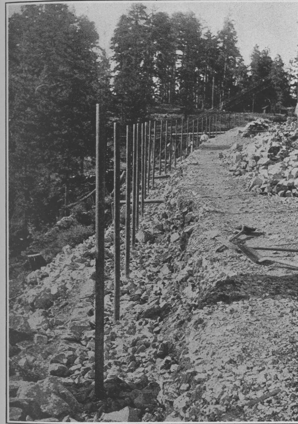
OTERO COUNTY. State Road No. 24. Sec. 4. Stone wall under construction. with 3-inch pipe imbedded in concrete for railing. Vicinity of Clouderoft; elevation 9,000 feet above sea level.
