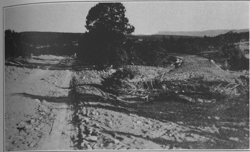
SAN MIGUEL COUNTY. State Road No. 1. Sec. 6. Showing old road to left and new construction and location to right.
