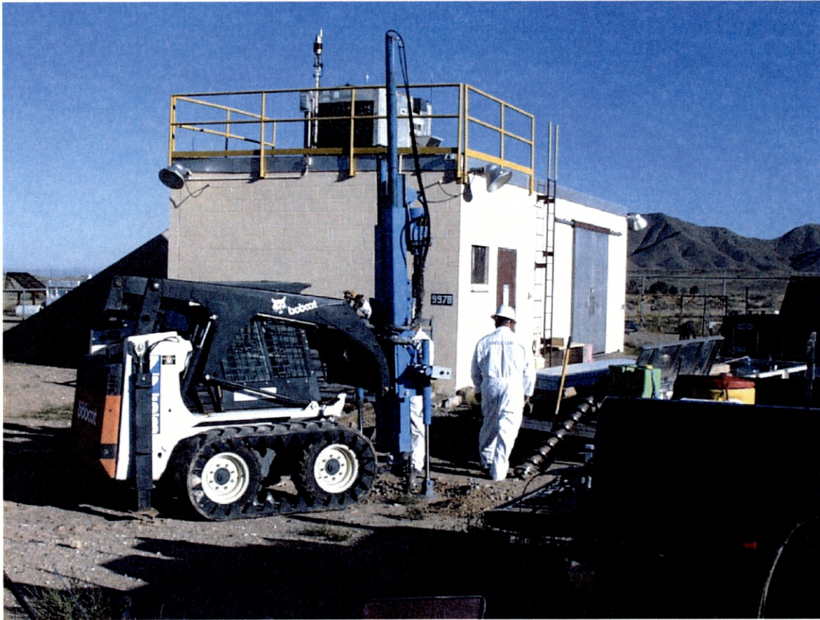
Figure 3.3-1 Collecting soil samples with the Geoprobe™ at DSS Site 1114, Building 9978 Drywell. View to the northwest. September 23, 2002
