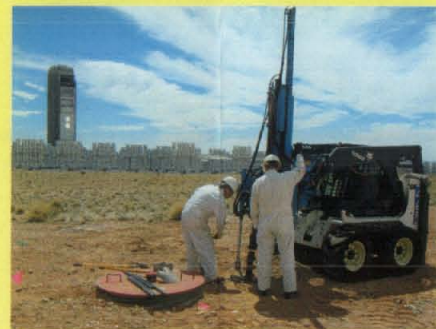
Collecting additional soil samples for VOCs from a borehole drilled adjacent to the seepage pit at AOC 1116 with the Solar Tower in background.
