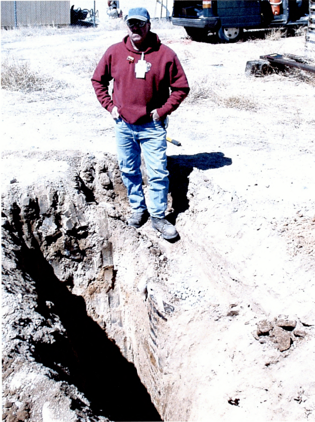
Figure 3.2-1 The metal culvert side of the drywell exposed during the backhoe excavation of the Building 9978 system. The base of the drywell was located at 5.5 feet below ground surface. View to the northwest. March 22, 2002
