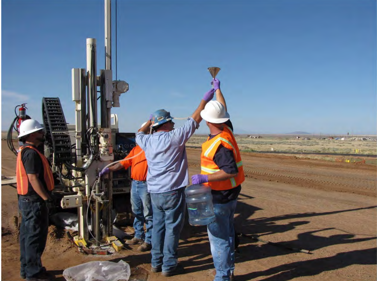
Figure 2-3 Hydrating the bentonite plug by pouring deionized water into tubing inserted into the Geoprobe rods at soil-vapor well MWL-SV01 location, August 7, 2009 (view to the southwest).
