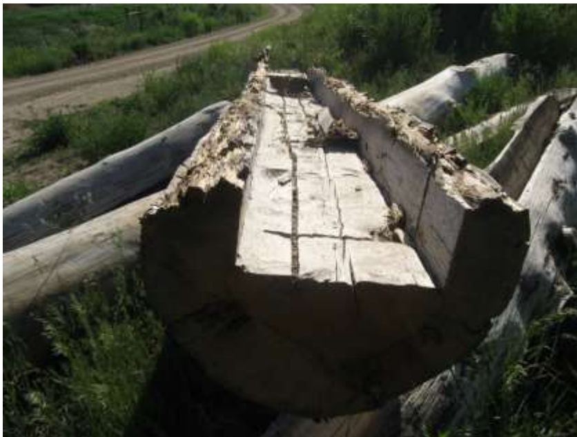
Wooden canoa at Las Trampas NM taken down for replacement. June 2008 Photo
