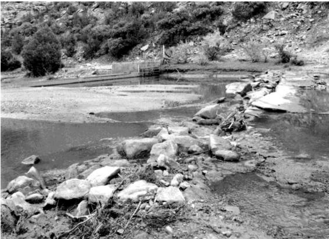
El Cerrito Remnant of Cement-Capped Brush and Rock Second Dam. Intake for Ditch at New Dam in Background. Sharon Stewart Photo June 2002
