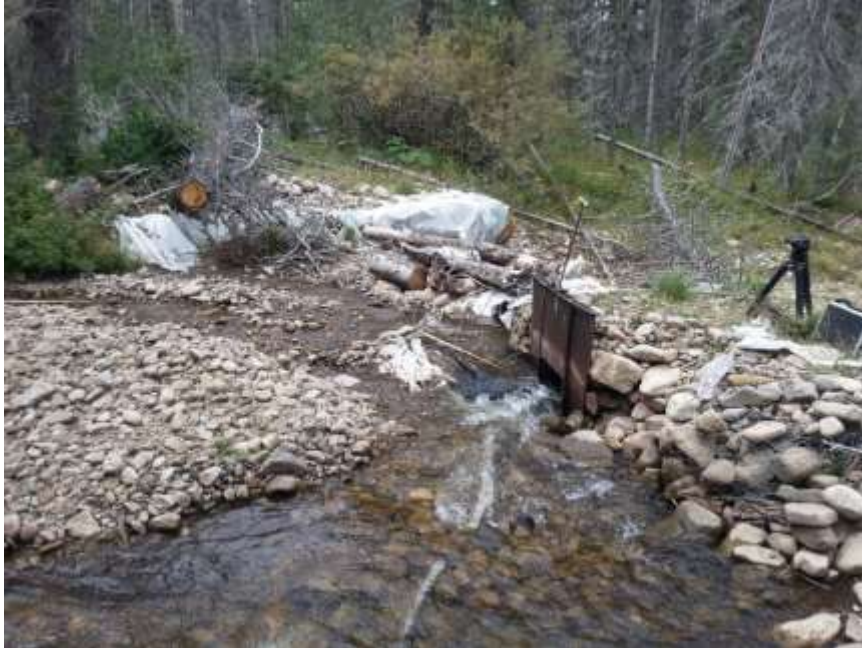
Encinal & Cañoncito Community Ditches Trans-Basin Diversion at Alamitos Creek before Modern Replacement. September 2017
