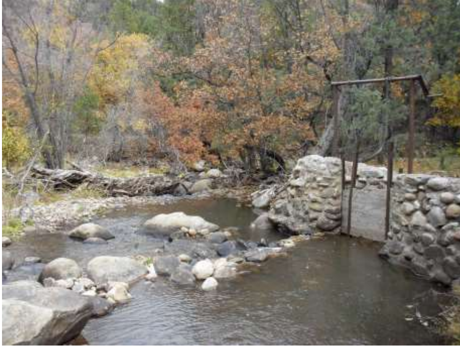
El Rito NM Presa of Stone Alignment & Chain Hoist Gate at Low Flow. October 2010
