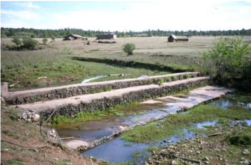
Rainsville Gabion Stone Wall with Concrete Cap on Río del Coyote near Mora NM. June 2001
