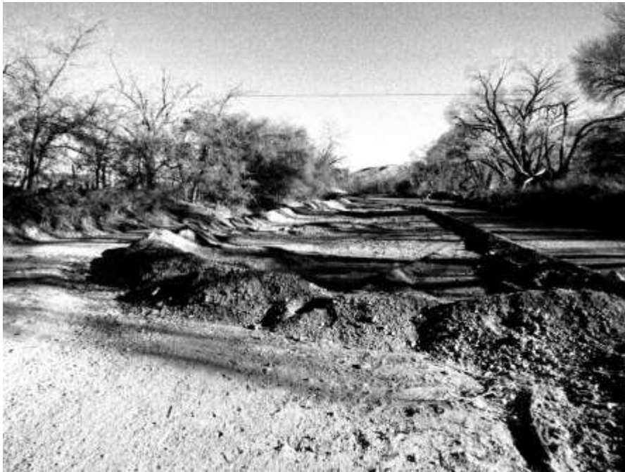
Monticello NM Earthen Push Up Dam on Alamosa Creek. Luis Pablo Martínez Photo March 2013
