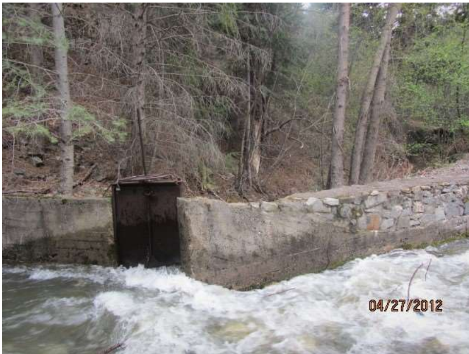
Río Hondo La Cuchilla Diversion at Valdez NM. Mortar and Stones. April 2012
