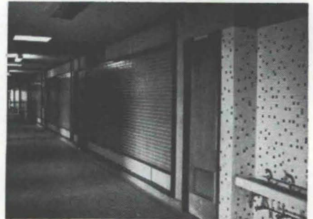
With CREST TILE-SET the completed job is finished in record time at considerable savings. And the client receives the performance, beauty and durability only ceramic tile offers.
