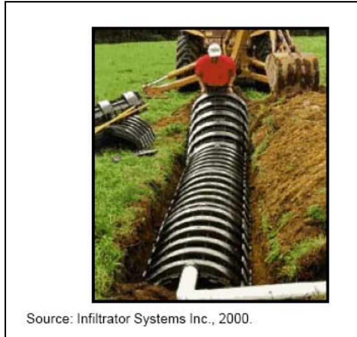
Figure 5: Gravelless Leaching Chamber
